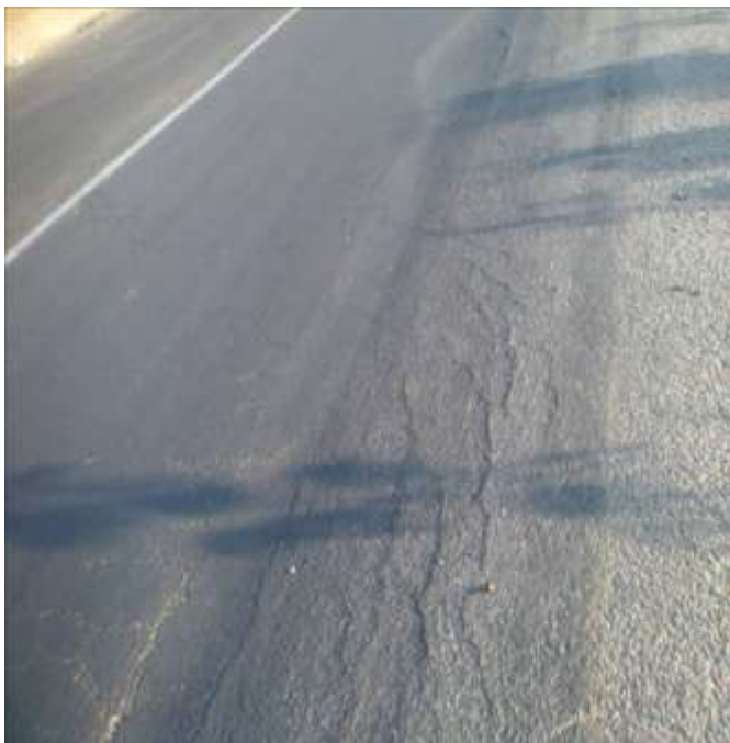
Fig.3. Typical rutting distress at site # 2 (Chainage 3+262)
