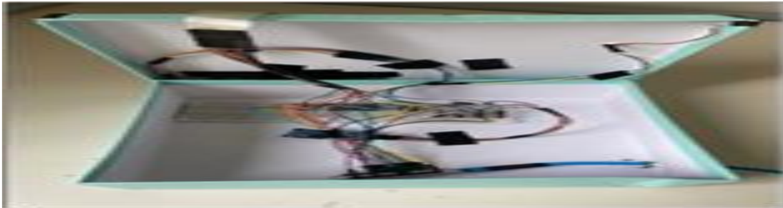
Figure 7. Hardware Development Setup (internal view)
