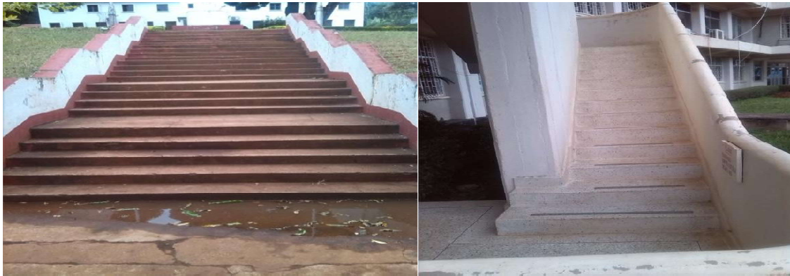
Unsupportive Infrastructures for Physically Disabled Leaners at Sampled public primary school
