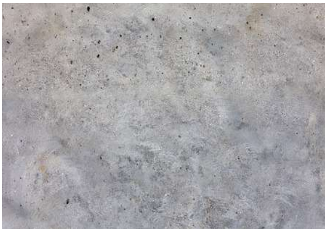
Figure 0.19: Example of wall texture inside the abandoned Penjara Pudu.
